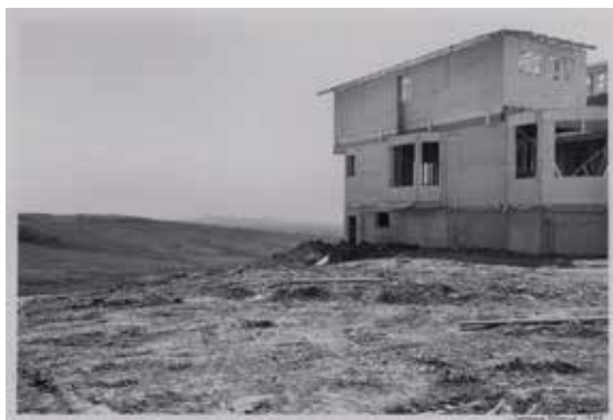
Jacques Rioux House Under Construction , 1985 Silver gelatin Collection of the Alberta Foundation for the Arts
